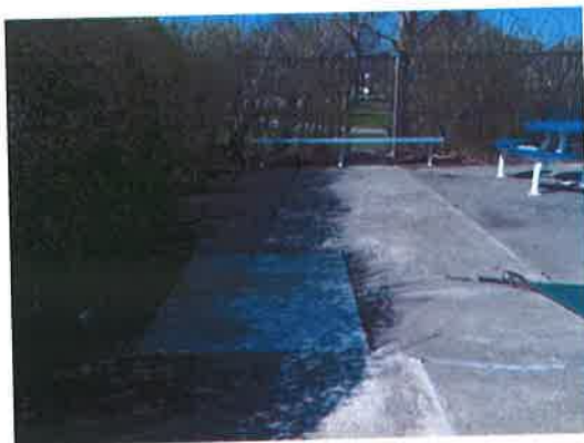
Planarity issues in concrete
