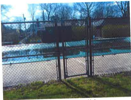
Fencing, poor condition
